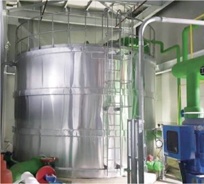
CONENSATE WATER TANK
