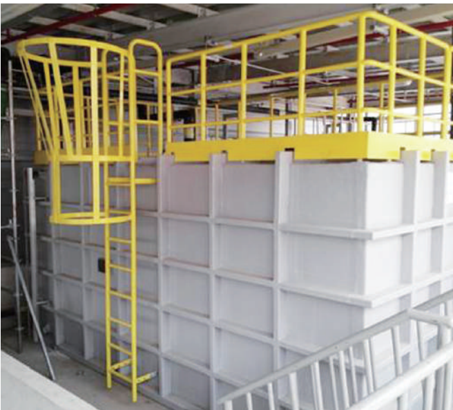
WASTE WATER TANK
