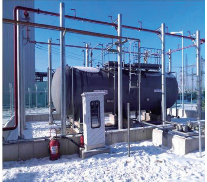
LUBE OIL TANK
