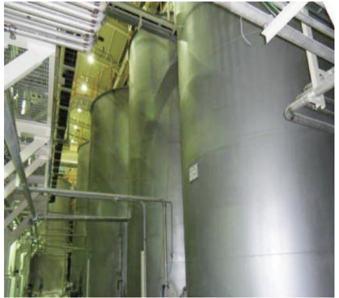
MILL DISCHARGE TANK
