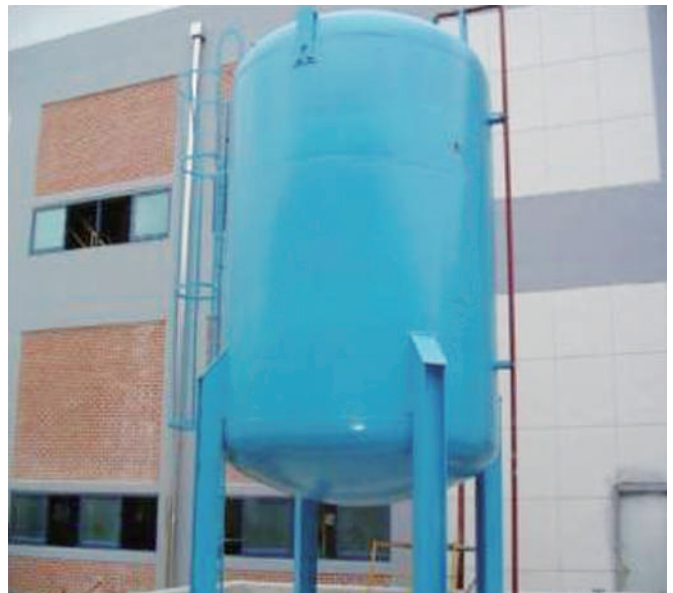
H 2 SO 4 TANK
