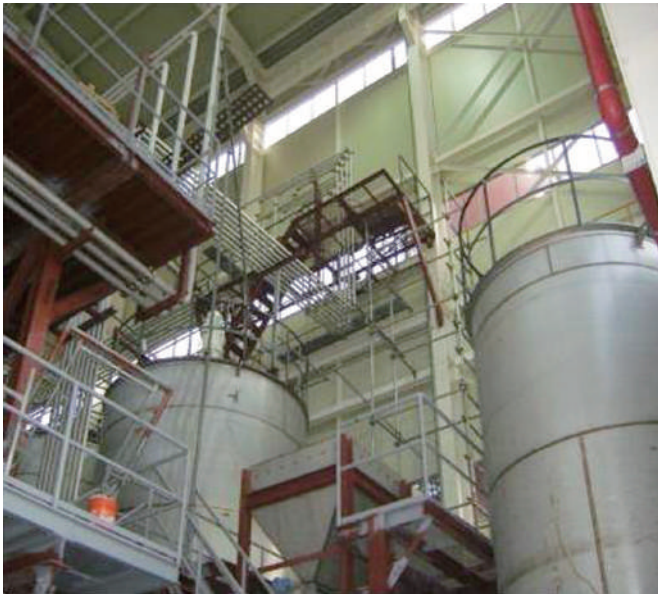
BIOCIDE STORAGE TANK
